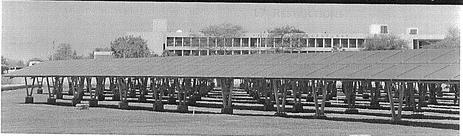
1 MW Multi-Technology PV Power Plant, Pandit Deendayal Petroleum University, Gandhinagar.
